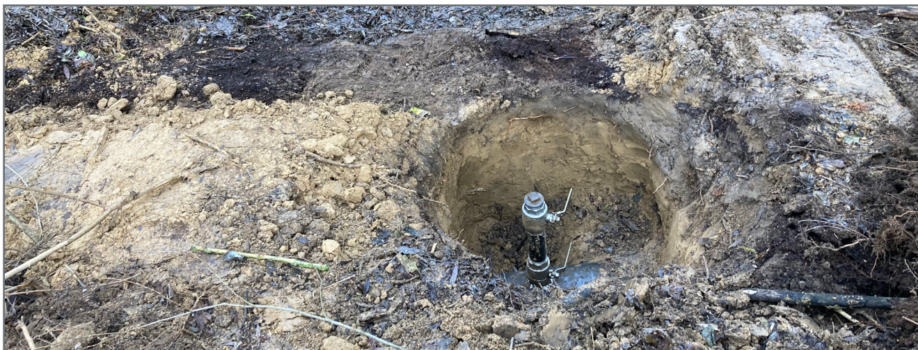
Figure 3: A tapping point located on TotalEnergies Marketing Belgium's pipeline
