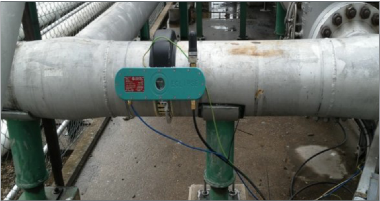
Figure 4: Atmos Eclipse installed on a section of the pipeline
