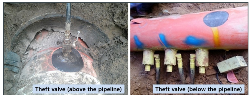
Figure 2: Small size hoses (1/2 inch) connected with oil pipeline for theft [3]
