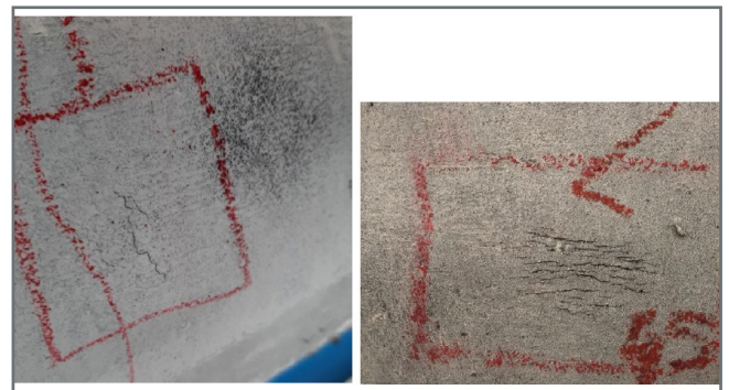
Figure 7: Circumferential and axial crack field SCC from TRAPIL field investigation
