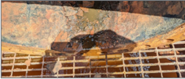
Figure 4: Scaling at 6 o'clock position
