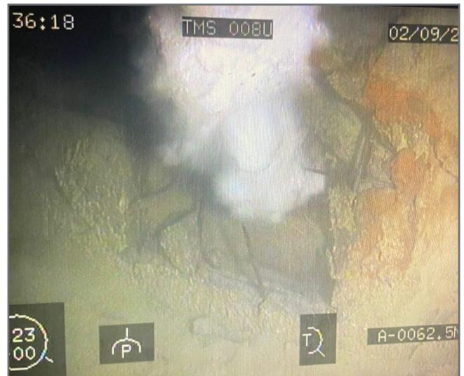
Figure 14: ROV Result on Second Damage of the Pipeline [5]
