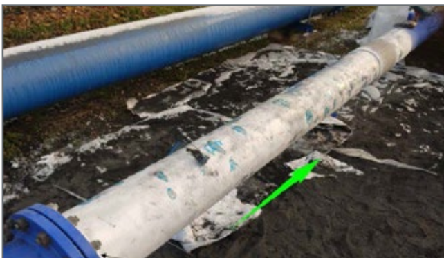
Figure 13 : Crack field pipeline section on Trapill's spool test
