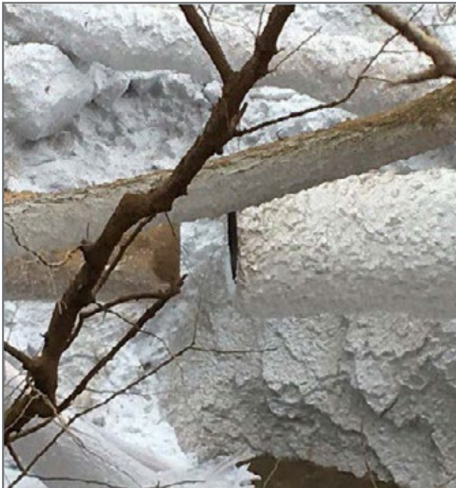
Figure 6: circumferential fatigue crack in a CO2 transport pipeline due to ground movements [6]
