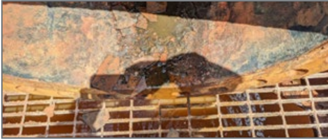
Figure 4: Scaling at 6 o'clock position
