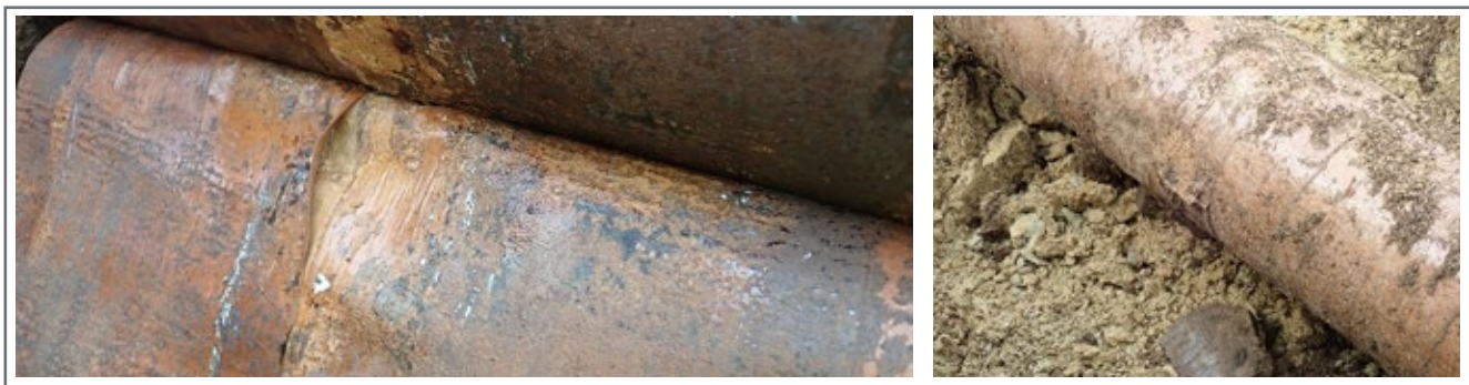
Figure 3: General findings at Location 1
