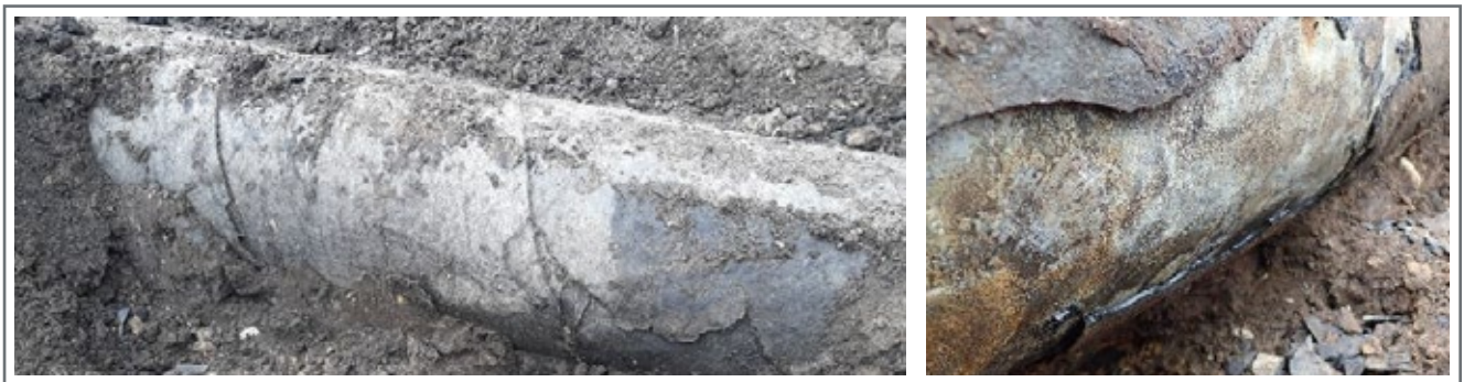
Figure 6: General findings at Location 4
