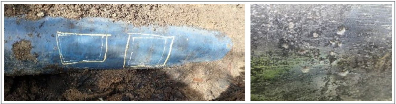
Figure 5: General findings at Location 3
