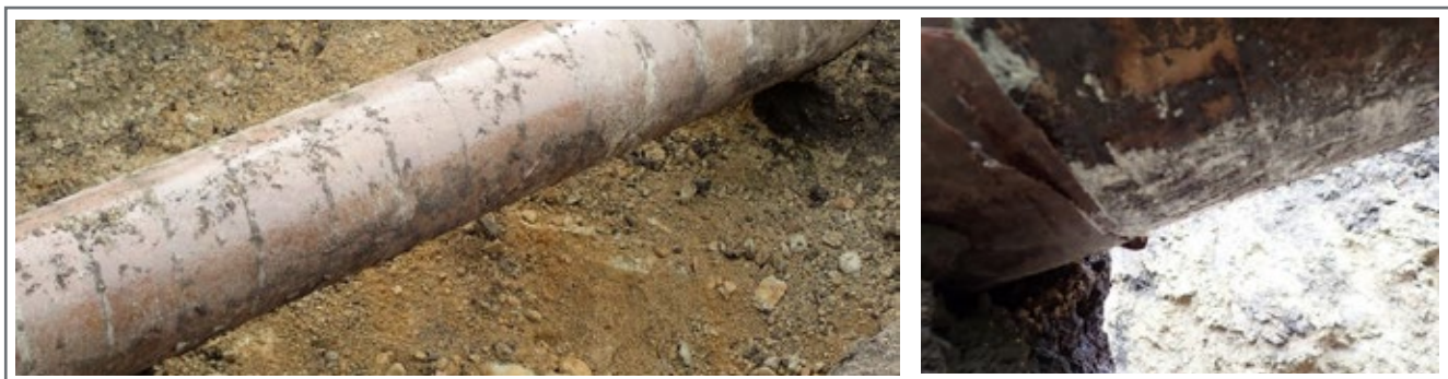
Figure 4: General findings at Location 2
