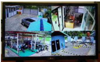
Figure 12. Monitoring Station by CCTV
