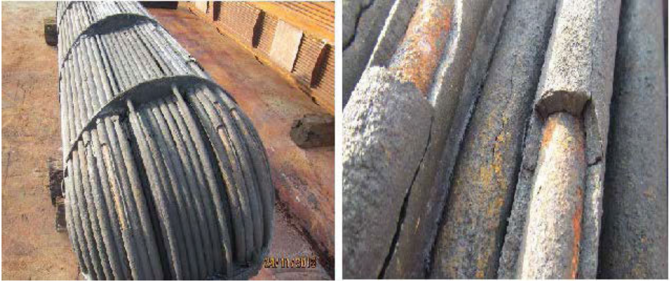
Figure 6. Severe scale build up on lean-rich MEG exchanger tubes
