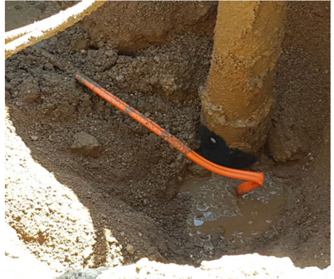
Figure 5 - A compromised conduit
